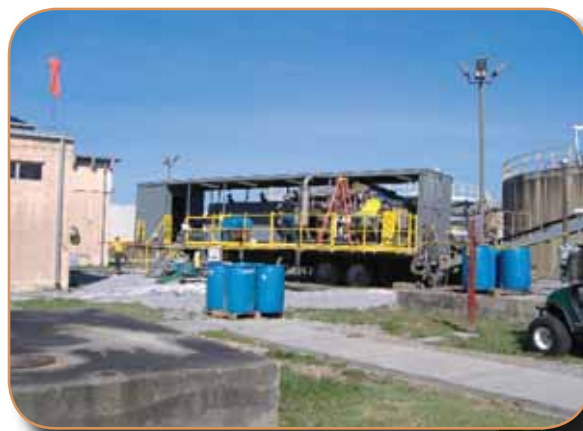
South Wastewater Treatment Plant
