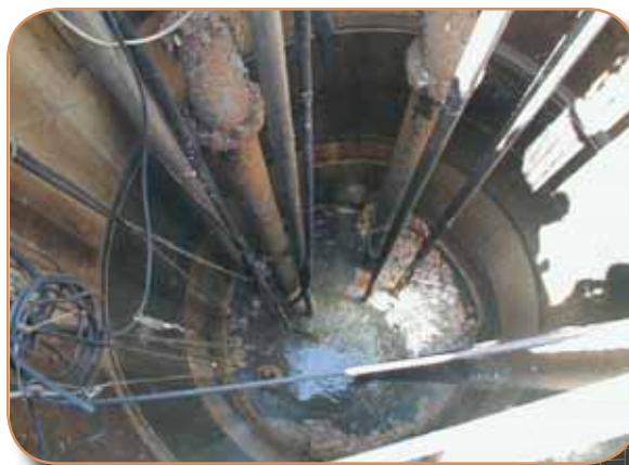
Pump Station Wet Well
