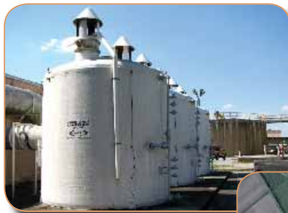
South Wastewater Treatment Plant
