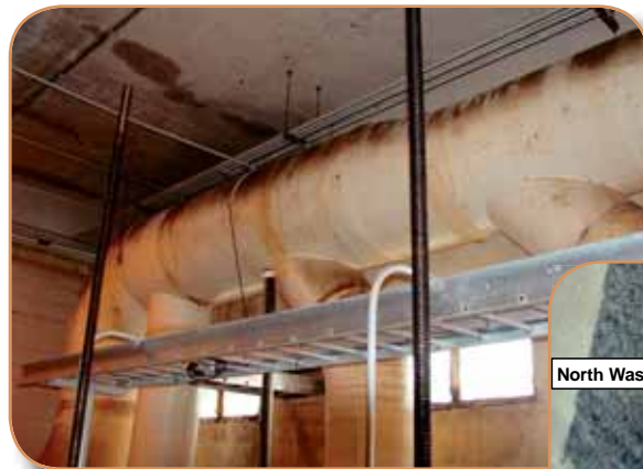
Ductwork in Gravity Main
