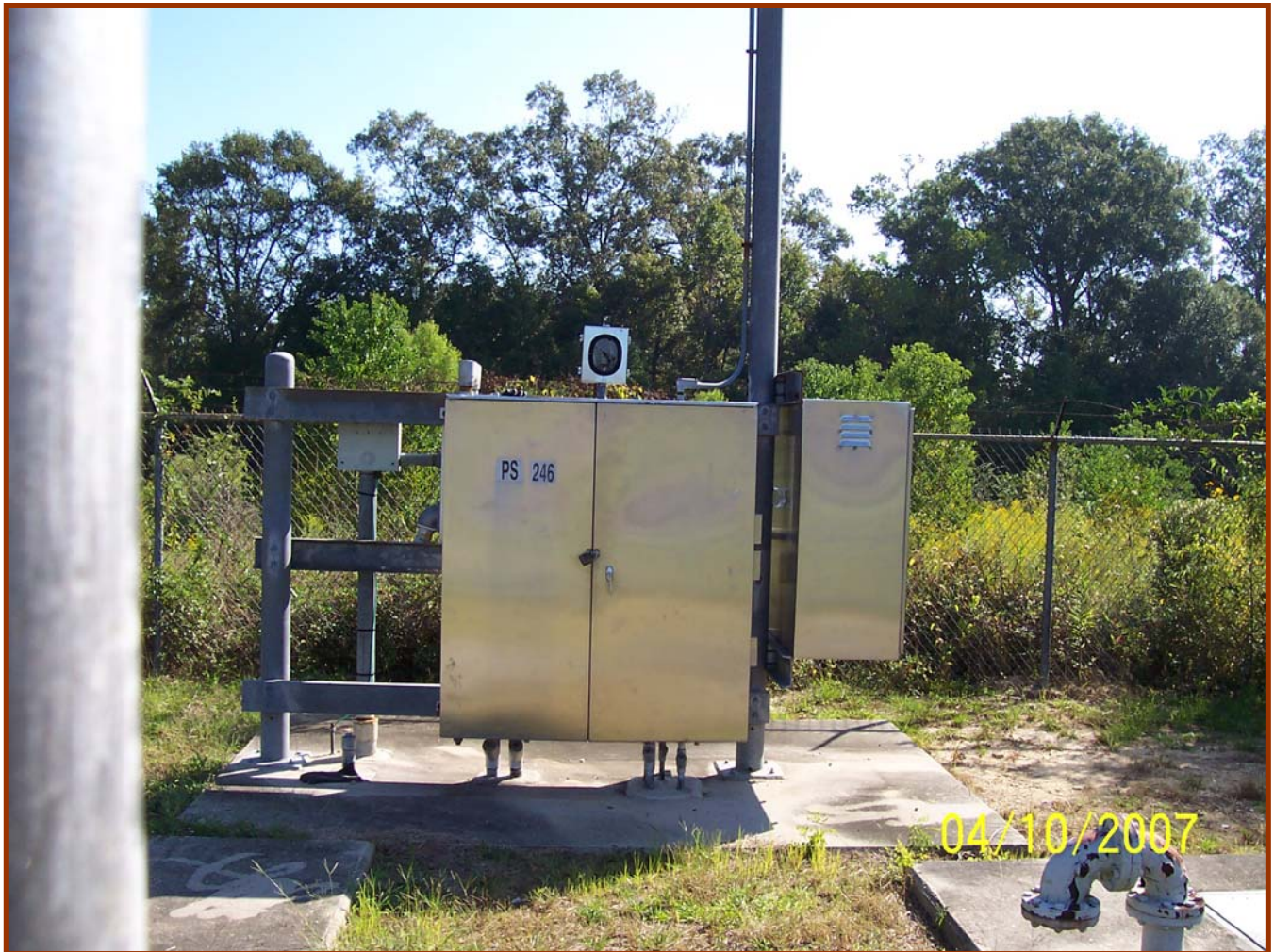
PS246 is located at the eastern end of Holly Fern Avenue, east of the intersection of Holly Fern Avenue and Green Gate Drive
