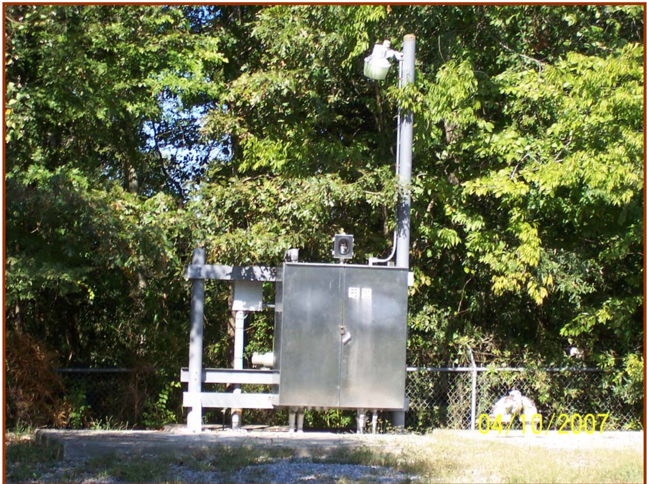
North Capacity Group Project 1A includes the replacement of PS150 which is located on North Park Avenue off of Northdale Drive
