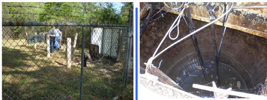
The Jefferson Highway/Highland Road Area Pump Station Improvements consists of various locations near Jefferson Highway, Highland Road, and Siegen Road. The project consists of capacity upgrades to Pump Stations 182, 223, 431, 327, 353, 278, 372, and 365.
