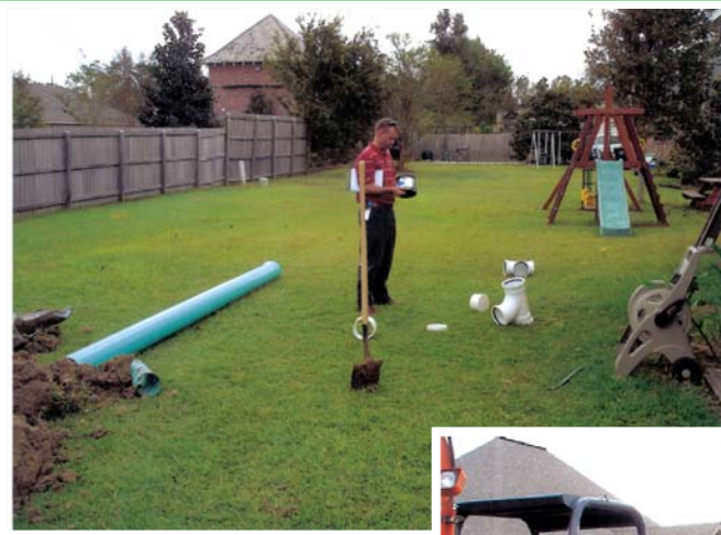
Rehabilitation Construction continues in the Jefferson Highway – Hoo Shoo Too Area project.
