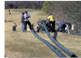
Preparations being made to join two sections of polyethylene pipe in the Kleinpeter Area.
