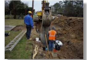
Bedding material is being installed along the forcemain in the Gurney Road – Joor Road project.
