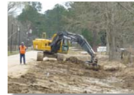
Rough grading an existing swale after pipeline installation along the Gurney Road – Joor Road project area.
