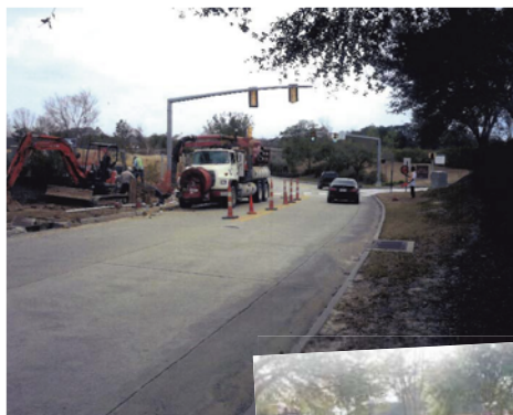
Near Pump Station 382, proper care is taken by the contractor when by-pass pumping started on the existing lift station.
