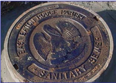
One of the first steps in rehabilitation includes a physical inspection of manholes and pipes to identify blockages.
