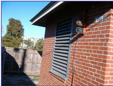
Pump Station #6, located on Stanford Avenue and Lakeshore Drive, will be upgraded.
