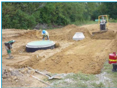
Wet wells and manholes are frequently upgraded during construction.
