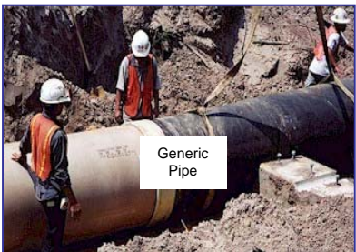
A total of 54,680 linear feet of various sizes of force main will be upgraded in the project area.
