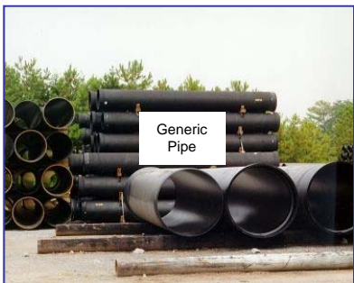
Approximately 450 linear feet of 12-inch gravity will be constructed in the project area.
