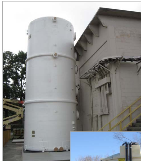
New biotower unit was installed at the force main headworks building.
