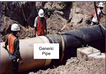
A total of 38,160 linear feet of force main will be constructed in the project area.
