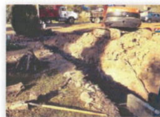
The project area consists of 117,110 linear feet of pipe to be rehabilitated.
