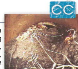
One of the first steps in rehabilitation includes a physical pipe inspection to identify blockages.
