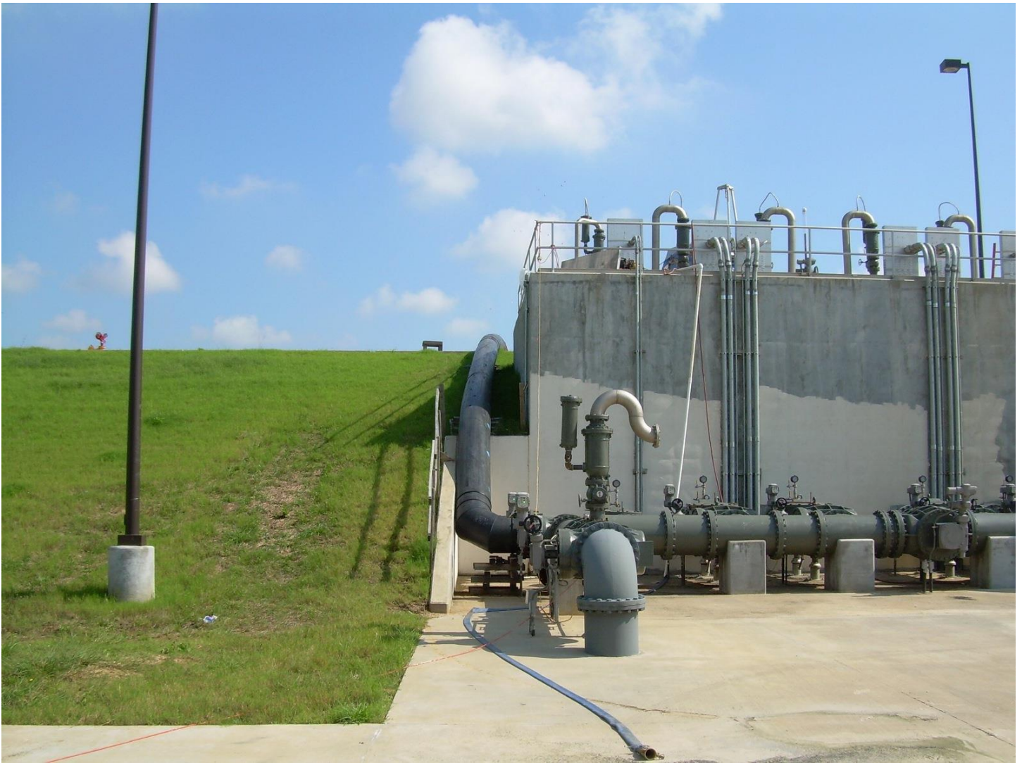
Figure 2. Temporary valves and recirculation above-ground HDPE piping installed to facilitate pump station testing
